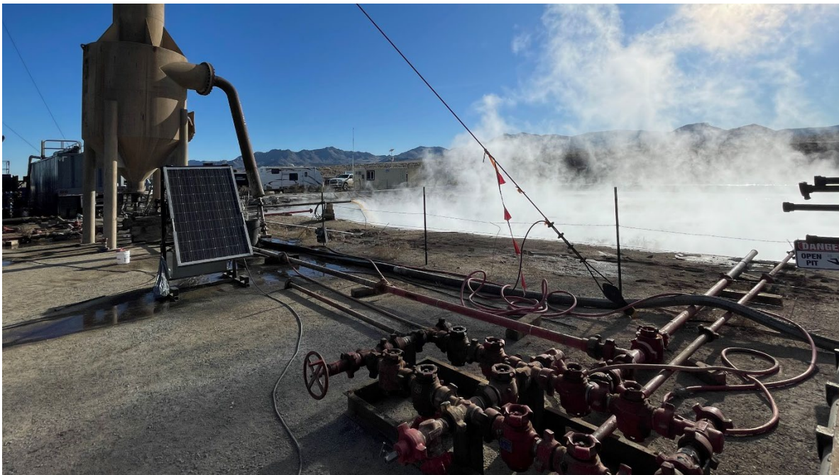
Figure B.3-4. Some of the flow equipment and instrumentation. The atmospheric separator and liquid flow line are shown in the background. A choke manifold (to control the flow rate from the well) is seen in the foreground.
