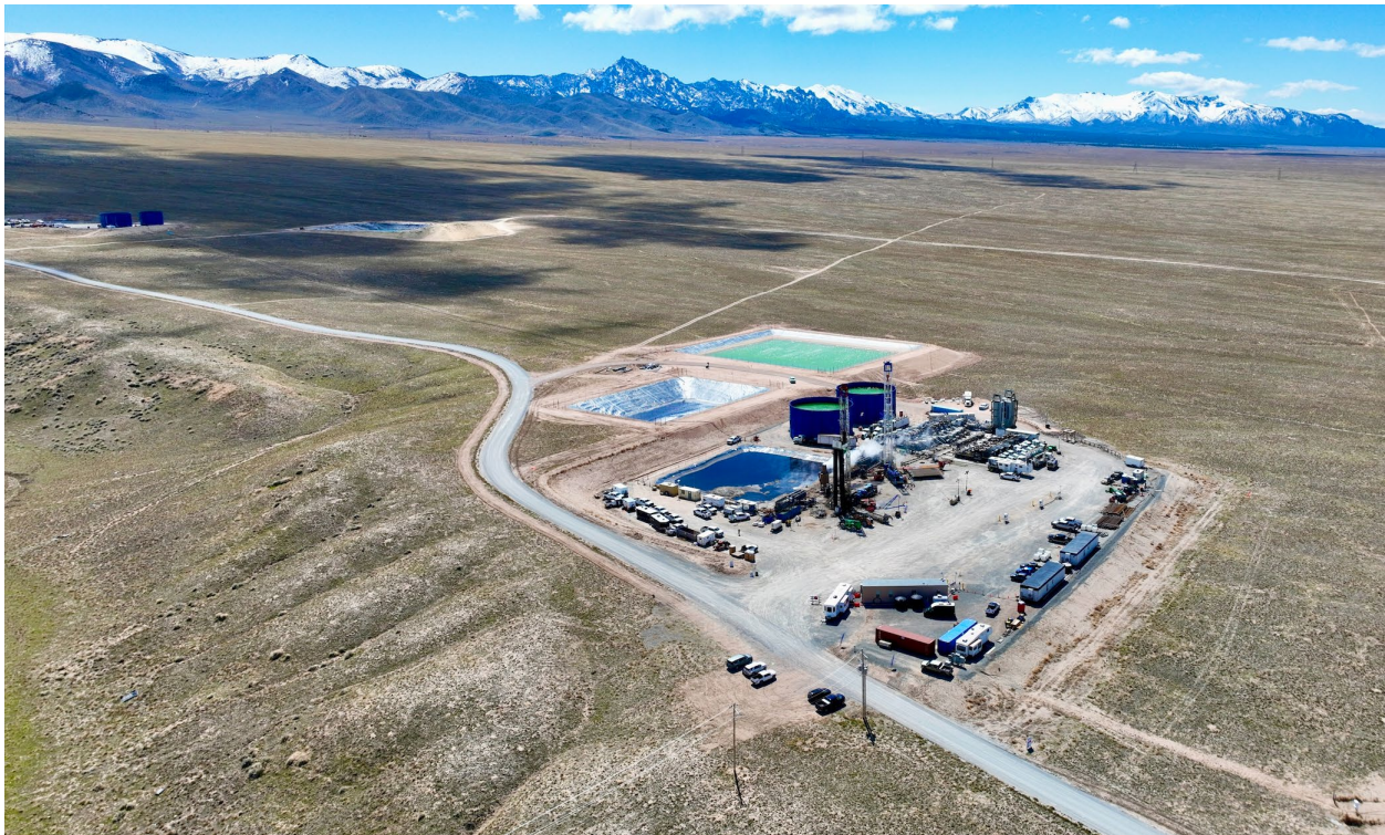
Figure A-1. Drone shot looking south taken during the stimulation of wells 16A/B(78)-32. The rigs are set up on the injection and production wells. The two large pits adjacent to the well pad hold a total of 200,000 barrels. They will provide water storage during future drilling, and stimulation and circulation testing. The pit in the upper left belongs to Fervo Energy.
